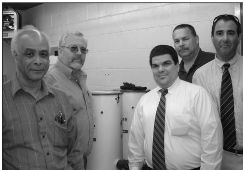
Westbury Water District Superintendent John R. Ingram (second from left) is joined by (left to right) Commissioners Kenneth O. Jones, Vincent Abbatiello and William C. Olson in checking on one of the utility's chlorinators. District Consulting Engineer William Merklin, of Dvirka and Bartilucci, also visited the well site.
