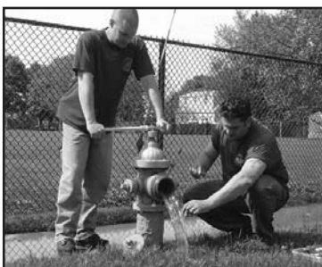
Westbury Water District employees Todd Weiss (left) and Matt Dinuzzo flush a hydrant and take a chlorine sample to insure a balanced chlorine residual in the distribution system.
