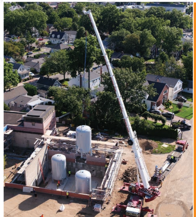
Aerial view of the Granular Activated Carbon (GAC) vessels being lowered into place.
